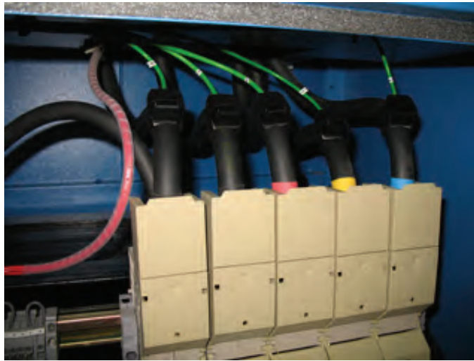
Exertherm Cable sensors installed
